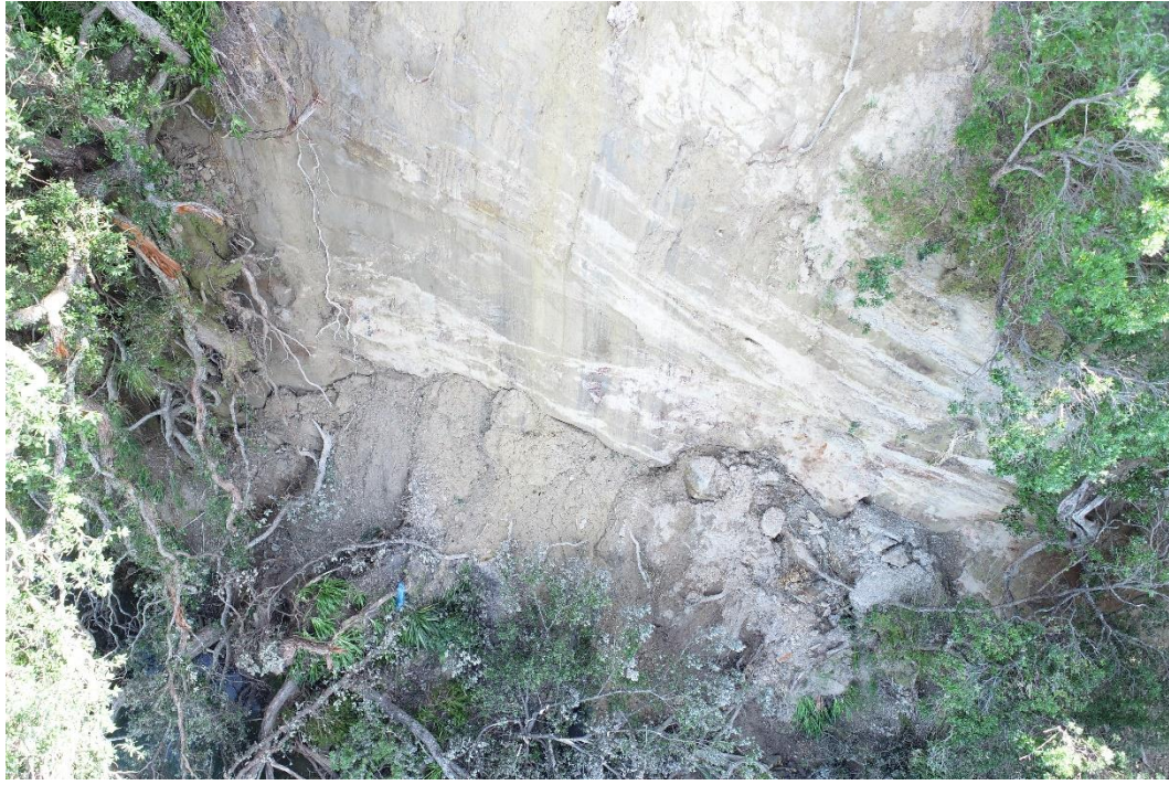
Slip 2 – Drone footage showing adjacent growth (for depth of slip) and debris
