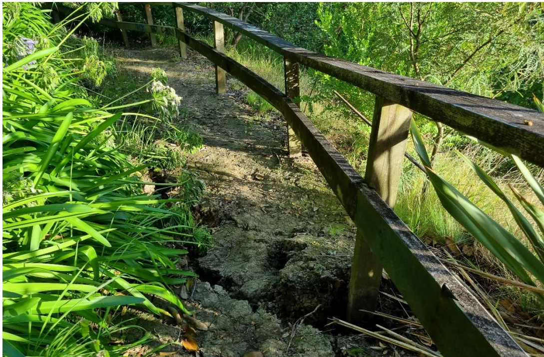
Slip 3 – Tension cracks on 9 February (prior to slip)
