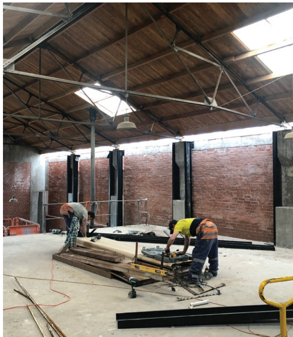
Milton Street Substation interior. Photo: Clark Mauger.
